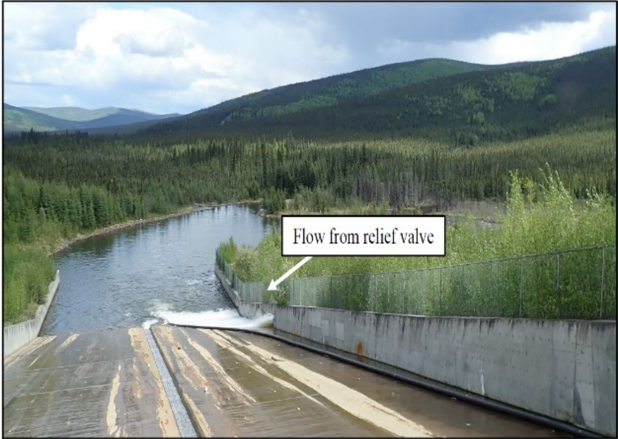
Figure 7. WSR relief valve open into spillway on June 4, 2021.
