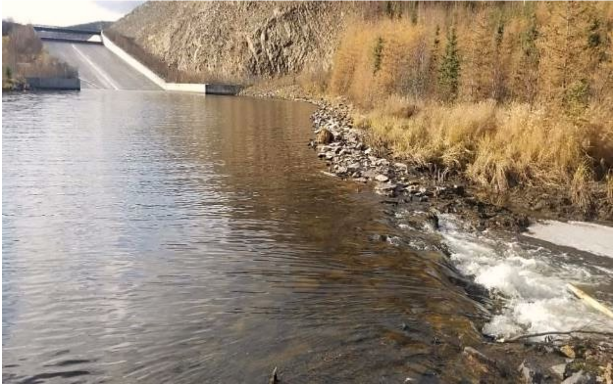
Figure 42. Fort Knox Stilling Basin outlet after part of the beaver dam was washed out, which lowered the water level by about two vertical feet.
