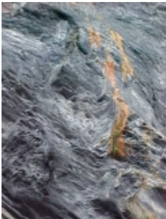
Pyritic Rock Iron Staining
