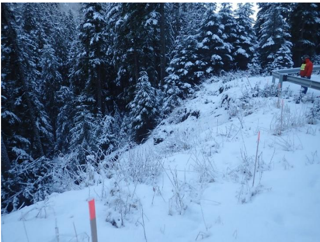
Photo 9. Crown (upper edge) of 7.5 mile landslide.
