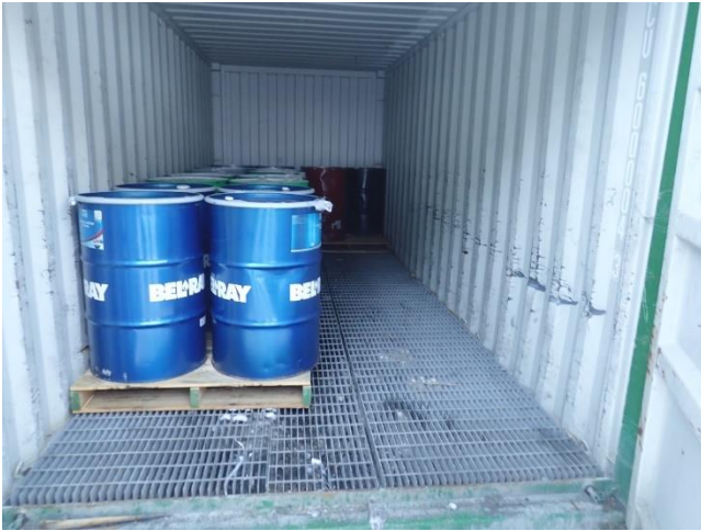
Photo 5. 920 warehouse storage container with appropriate secondary containment.
