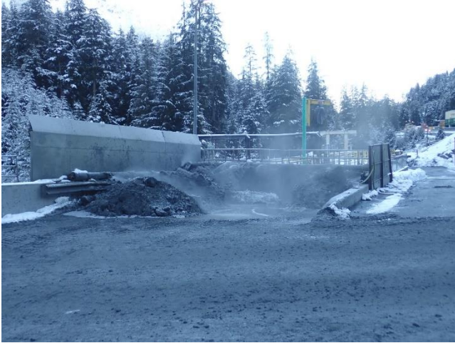
Photo 4. Degrit basin DB01.
