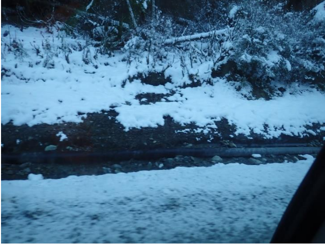
Photo 19. Pipes exposed in B-road ditch due to December storm erosion.
