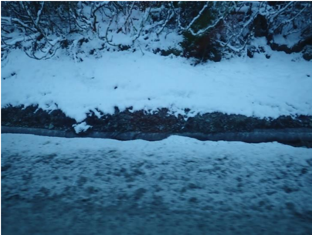
Photo 20. Pipes exposed in B-road ditch due to December storm erosion.
