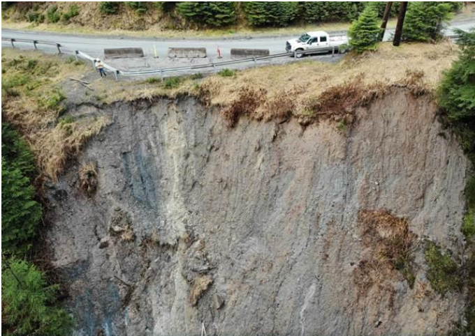
Photo 11. Photo provided by HGCMC on December 9, 2020. 7.5 mile landslide below B-road.
