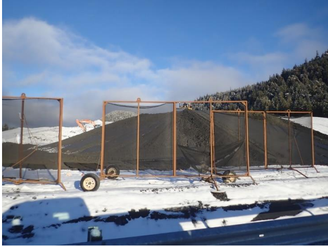
Photo 25. Tailings being placed in S3P1 area with fugitive dust control screens in place.
