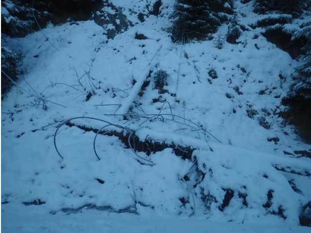
Photo 13. Cables on the ground adjacent to the B-road due to storm impacts.
