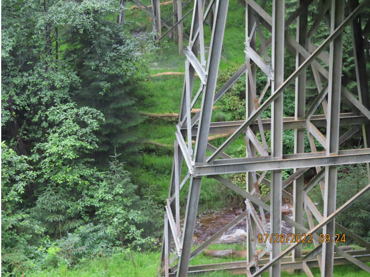
Photo 15. Downhill side Zinc Creek Bridge abutment showing recently replaced wattles and substantial vegetation growth.
