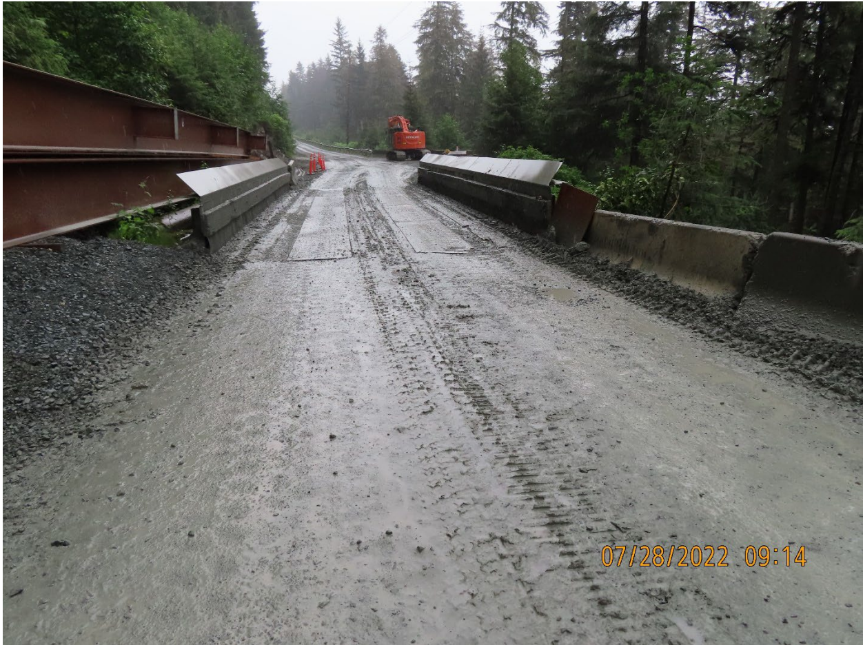
Photo 13. Downhill side of the Falls Creek Bridge. Plywood used on the right of the photo, and a coarse-grained fill berm on the left of the photo, preventing sediment from reaching the abutment from the roadway. These features will be improved with bridge replacement scheduled to begin August 10, 2022.
