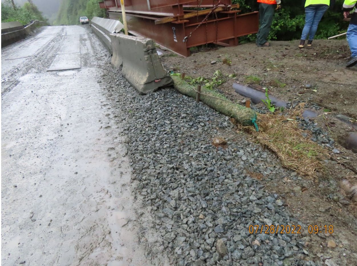
Photo 14. Temporary sediment deflection wattles and concrete barrier on the uphill side of the Falls Creek Bridge. Steel girders to be used in bridge replacement scheduled to begin August 10, 2022, are visible to the right of the bridge.
