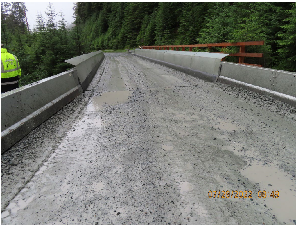
Photo 6. Killer Creek Bridge, showing effective sediment deflection barriers at the uphill end.
