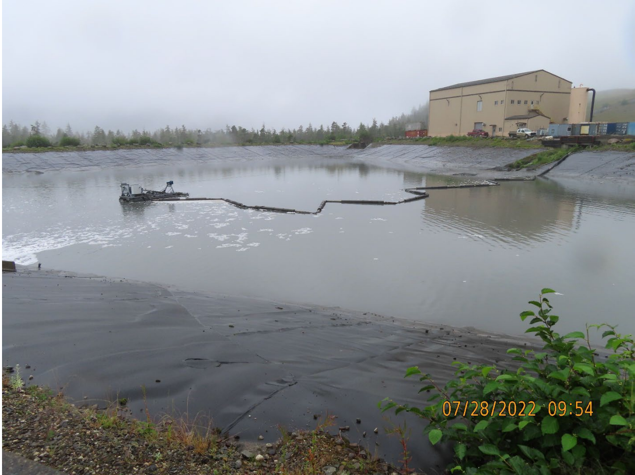
Photo 21. Pond 7 receiving contact and process water. Dredge in photograph was not actively operating.
