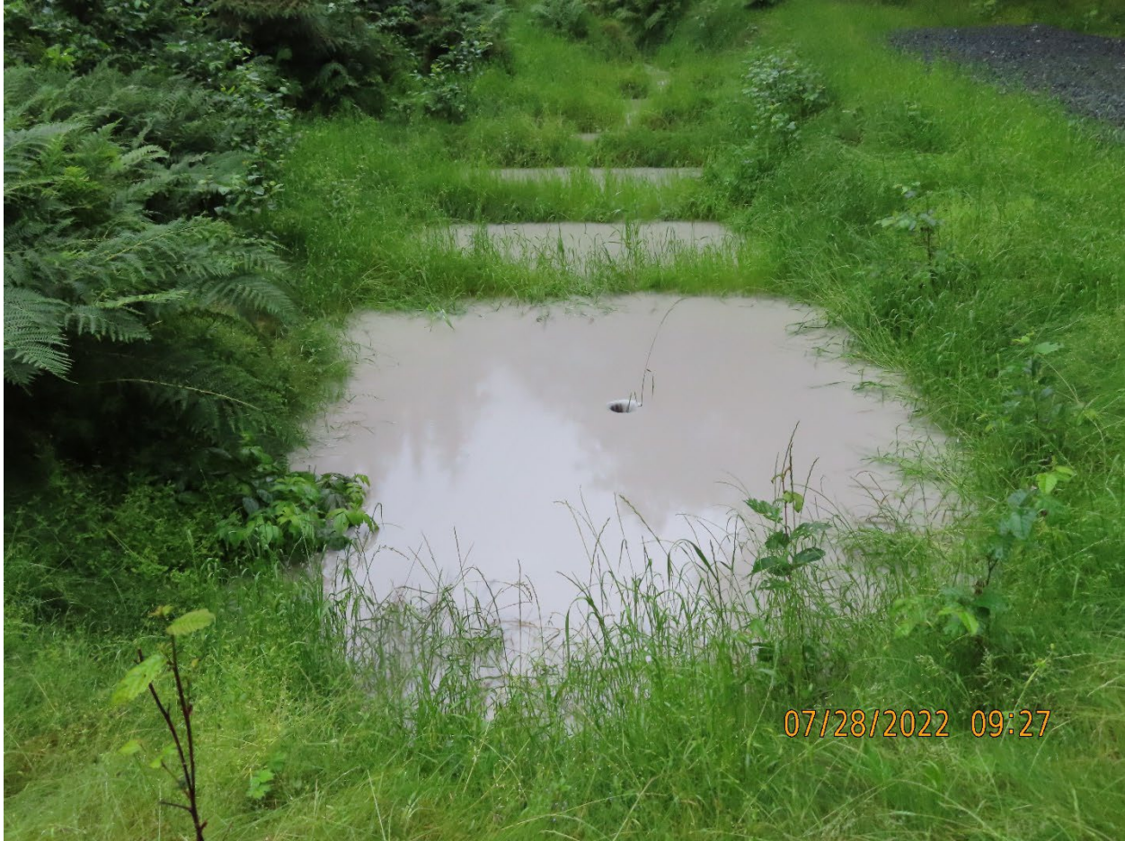
Photo 17. B-Road Stormwater BMP located uphill from the Zinc Creek Bridge. Downpipe that leads to discharge pipe visible at center of lower sump.
