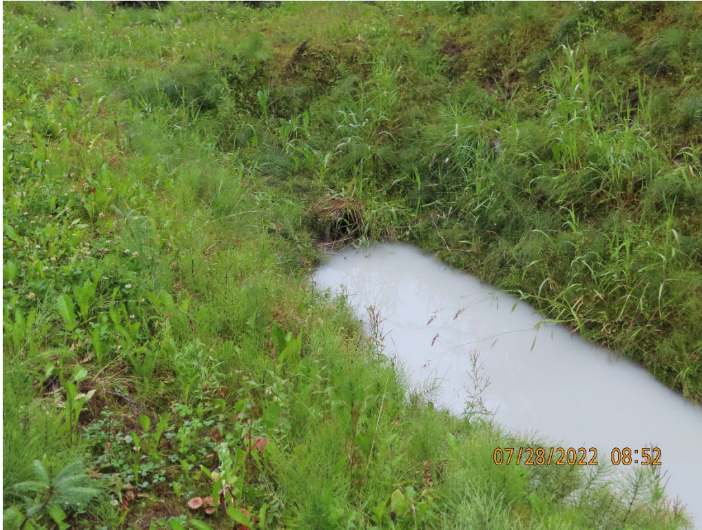
Photo 9. Stormwater BMP at the uphill end of Killer Creek Bridge from which sediment has been removed to restore sediment settling function.
