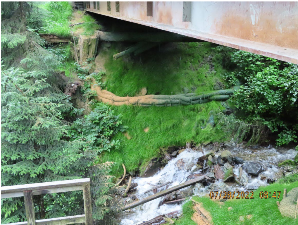
Photo 8. Downhill side abutment BMPs at Killer Creek Bridge, showing new wattles and successful revegetation efforts.
