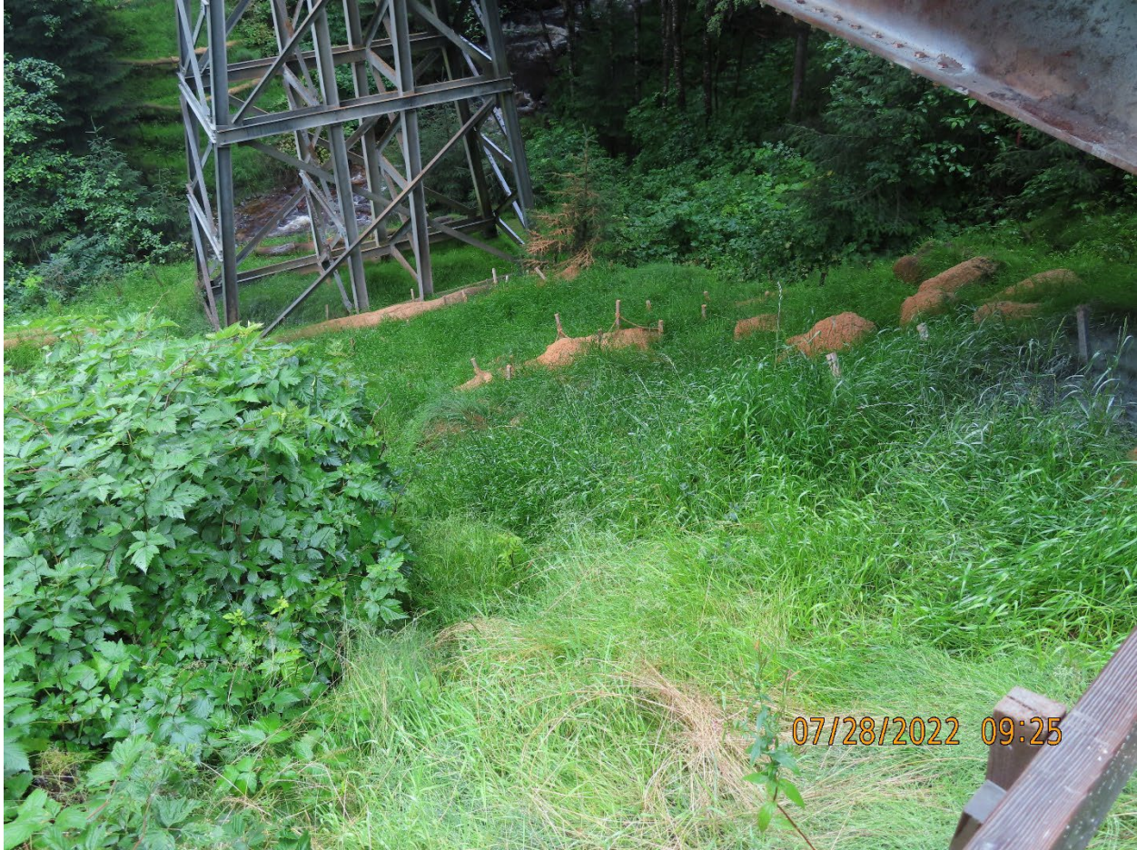
Photo 16. Uphill side Zinc Creek Bridge abutment showing recently replaced wattles and substantial vegetation growth.
