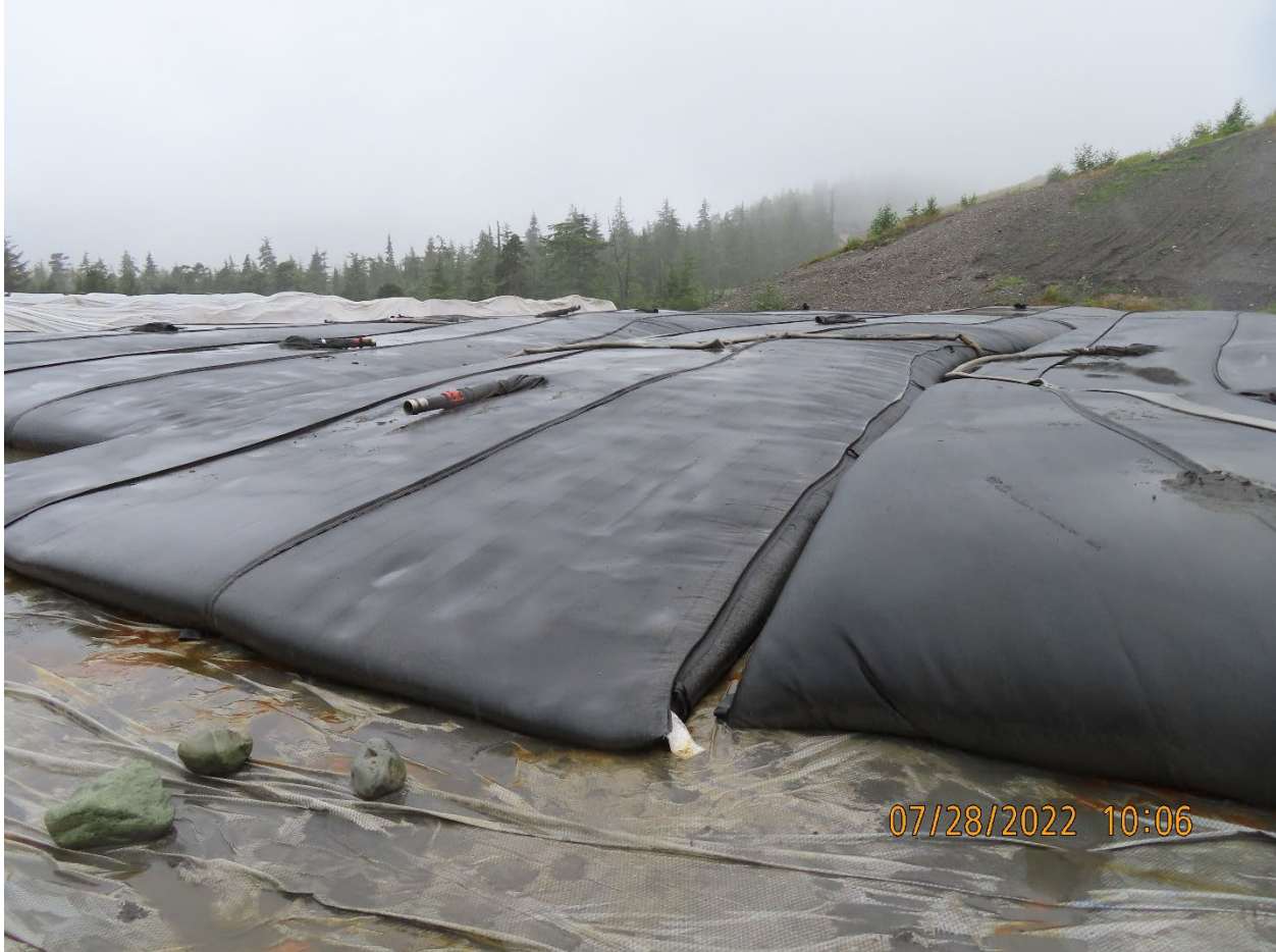
Photo 20. Dewatering bags containing sediment dredged from Pond 7. Located in the TDF east of the water treatment plant.
