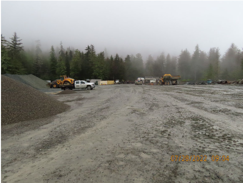
Photo 10. South end of Site E, used for equipment laydown and material storage.
