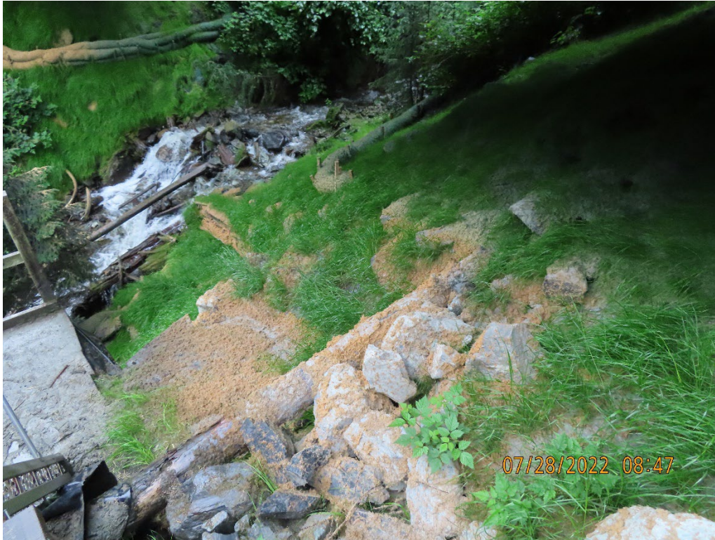
Photo 7. Uphill side BMPs at Killer Creek Bridge, showing new wattles and successful revegetation efforts.
