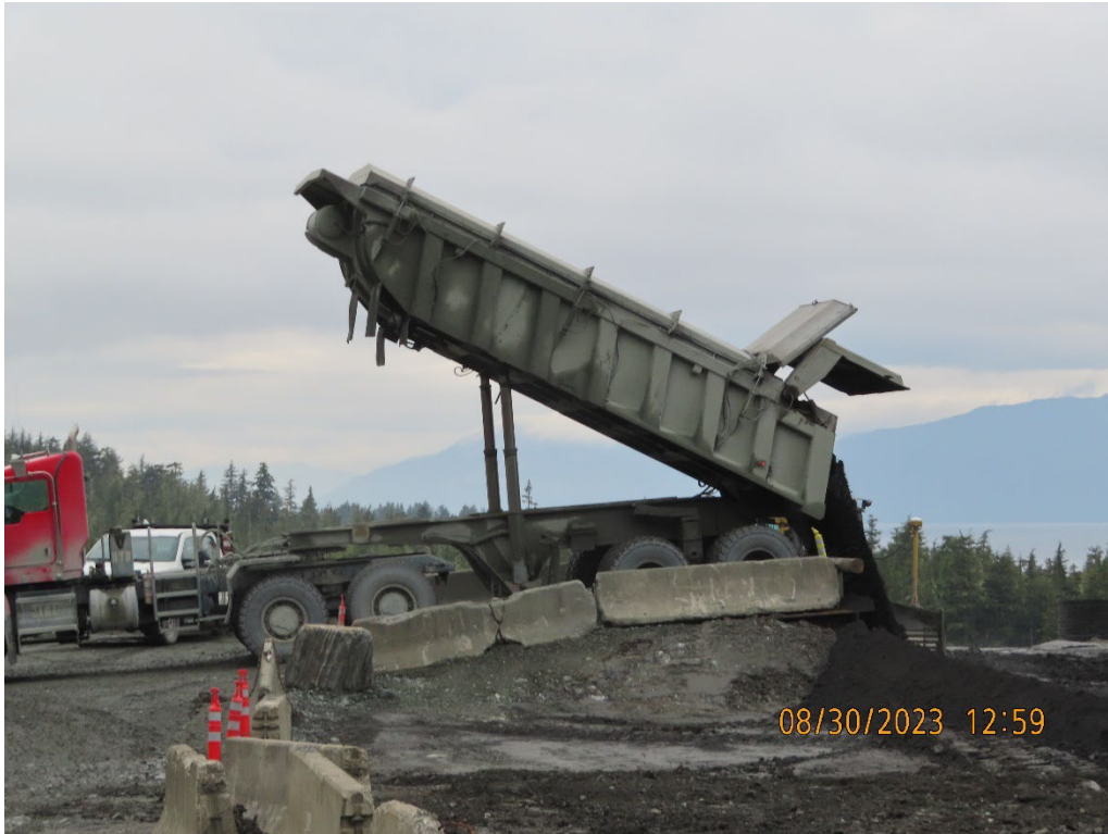
Photo 10. Max haul depositing tailings in the western section of the S3P1 TDF.
