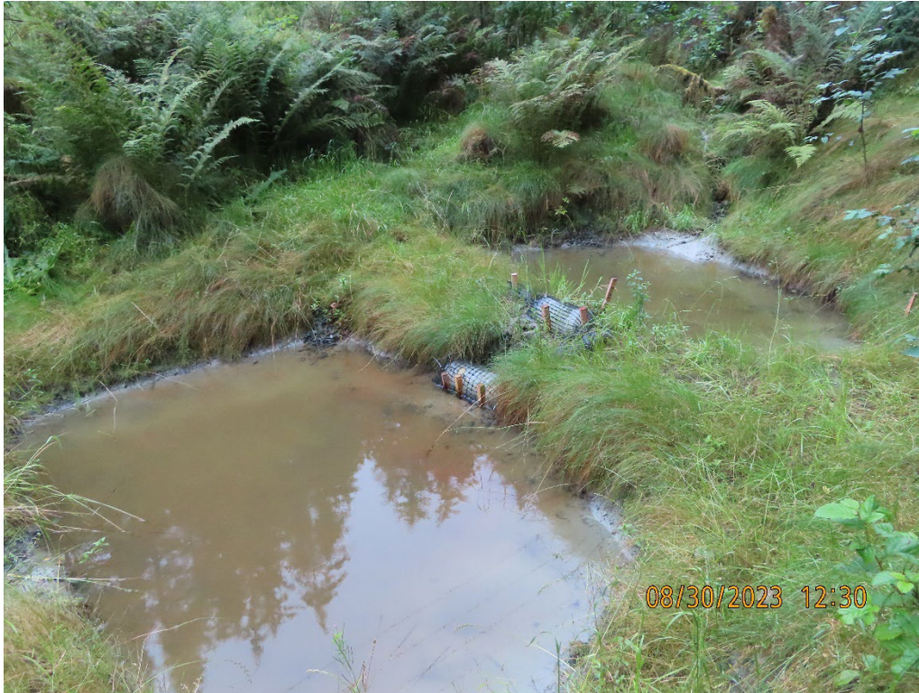
Photo 9. Zinc Creek Bridge abutment sediment ponds with Flocculant logs stage at the inlet of the first pond.
