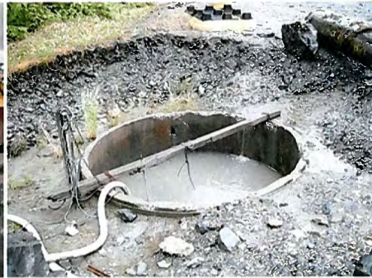
Contact water sump
