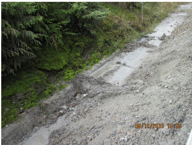
Photo 15. Rock check dams and sumps need improvements.
