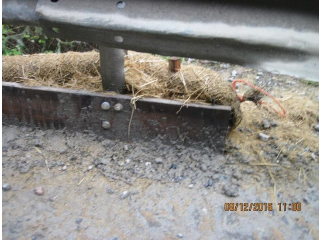
Photo 13. One temporary barrier was installed to monitor sediments accumulating on the downstream (camp side) of the Killer Creek bridge.
