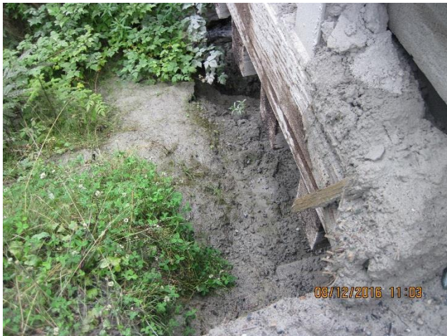
Photo 14. A barrier is needed to prevent sediment deposition on the downstream (Mill side) of the Falls Creek bridge.
