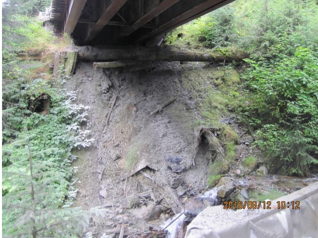
Photo 10. A liner (camp side of bridge) is not effectively preventing sediments from entering Killer Creek.
