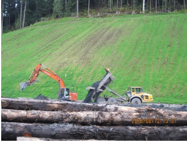
Photo 28. Blue/gray clay deposited on the perimeter of the pit.
