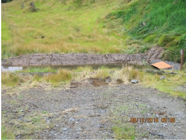
Photo 1. 1350 area trench and caisson for stormwater runoff from an old waste rock stockpile.
