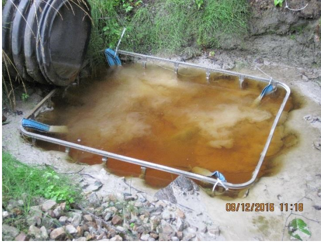
Photo 16. 3.1 mile B-road removable sediment screen.
