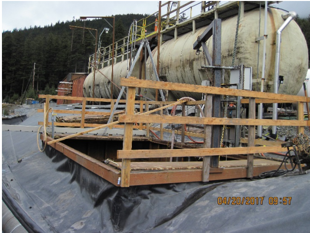
Photo 06. 920 sewage lift station.
