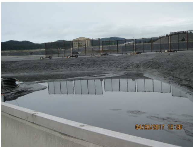
Photo 11. TDF wind fencing.
