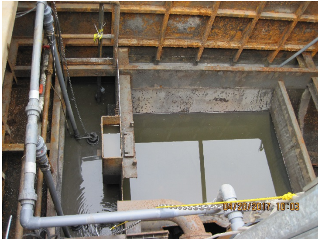
Photo 07. 920 sewage lift station.
