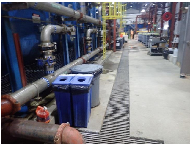
Photo 26. The TTF water treatment plant.
