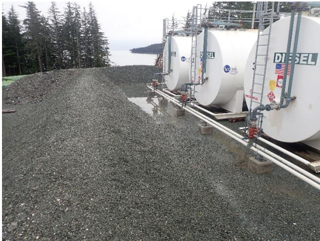
Photo 28. The fuel depot.
