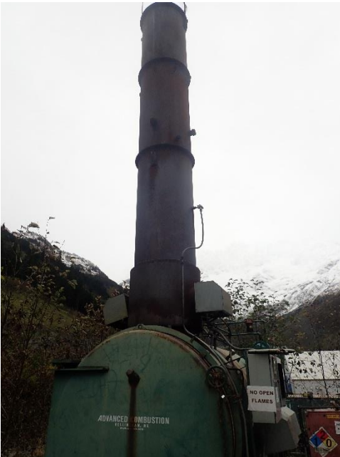
Photo 17. Coeur Alaska's solid waste incinerator.
