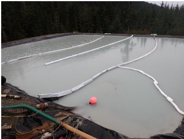
Photo 2. The CWTP's Pond 1.
