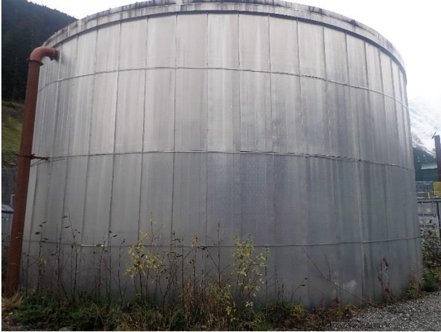
Photo 16. The firewater tank staged near the mill.
