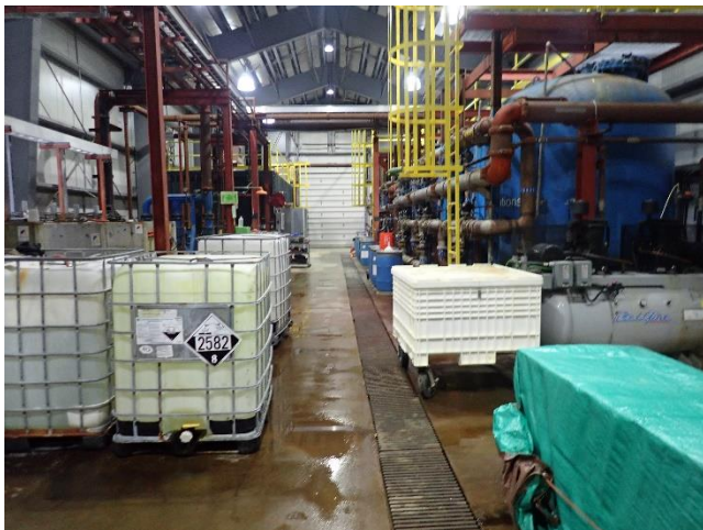
Photo 17. The TTF water treatment plant.
