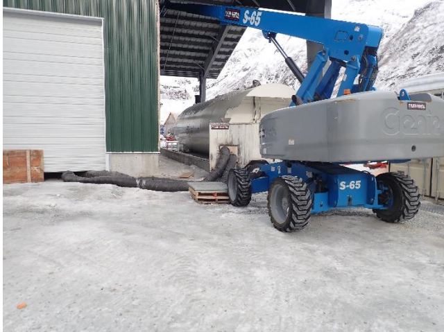
Photo 10. The 30,000-gallon day tank.
