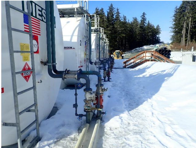
Photo 19. The fuel depot.
