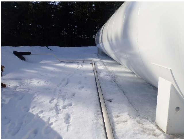
Photo 20. Snow and ice covering the tanks farms structural gravel pad.
