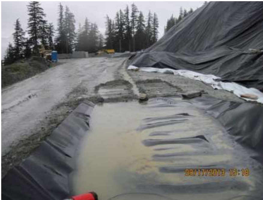
Photo 11. Drainage from the storage cells at pit 7 is directed to the sump in the foreground.
