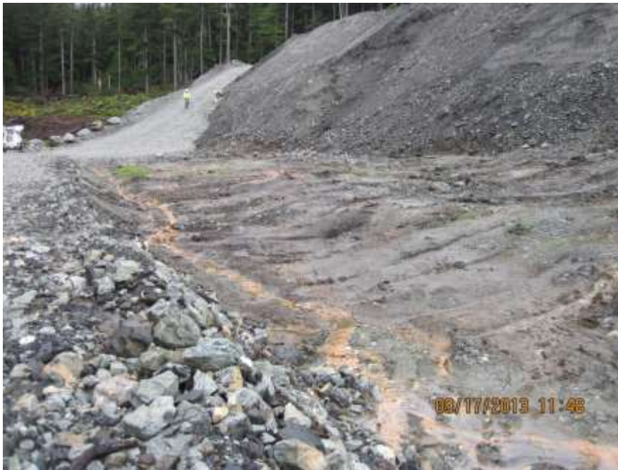
Photo 04. Acid rock drainage is still occurring at the base of the site where the graphitic phyllite was excavated.
