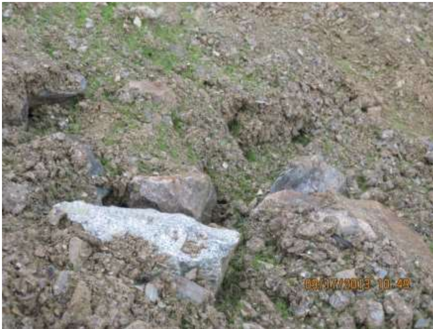
Photo 02. Some erosion is occurring in the biopolymer test plot where the subgrade has become exposed.
