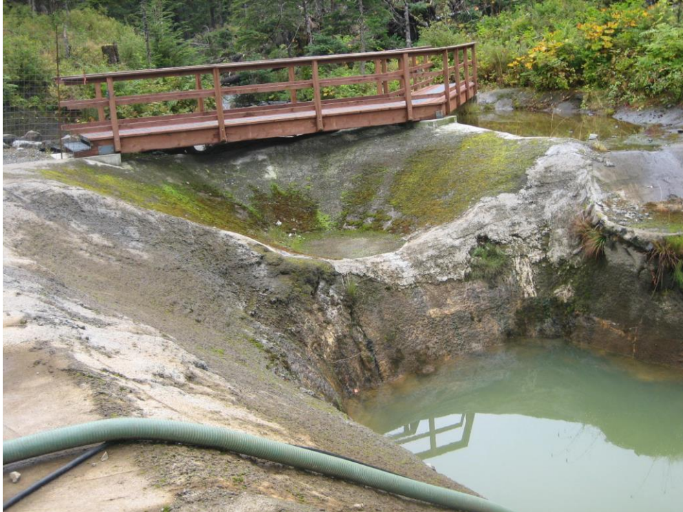
Photo EE Lower Slate Lake Dam collection channel and sump along and downstream of west groin of dam below shotcreted west abutment wall.
