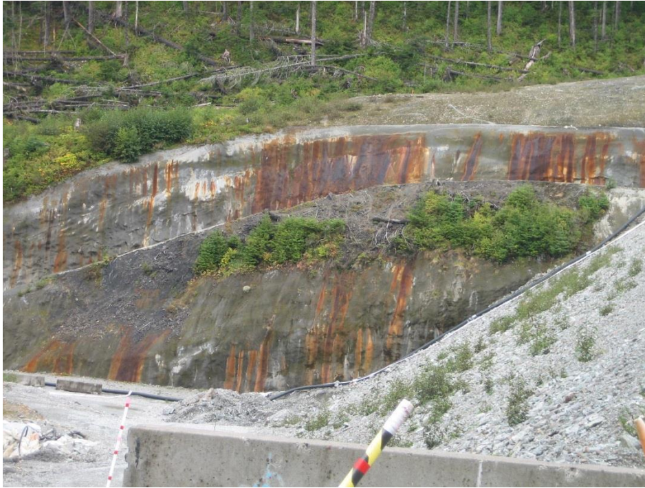
Photo Q Stage 2 Interim Spillway west wall and west abutment wall below spillway and downstream of Stage 2 Dam toe, shotcrete spillway walls with ARD seepage staining on spillway & abutment walls, looking west.
