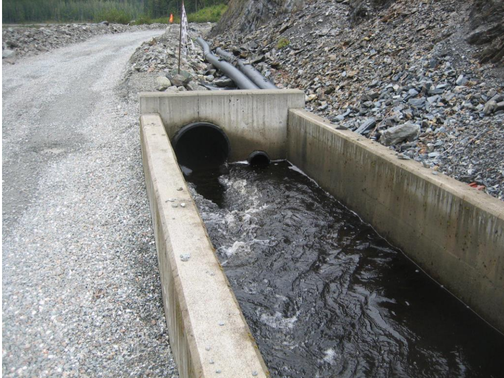
Photo M Parshall Flume for combined flow from Lower Slate Creek Diversion Dam & North Diversions at east (left) abutment of dam
