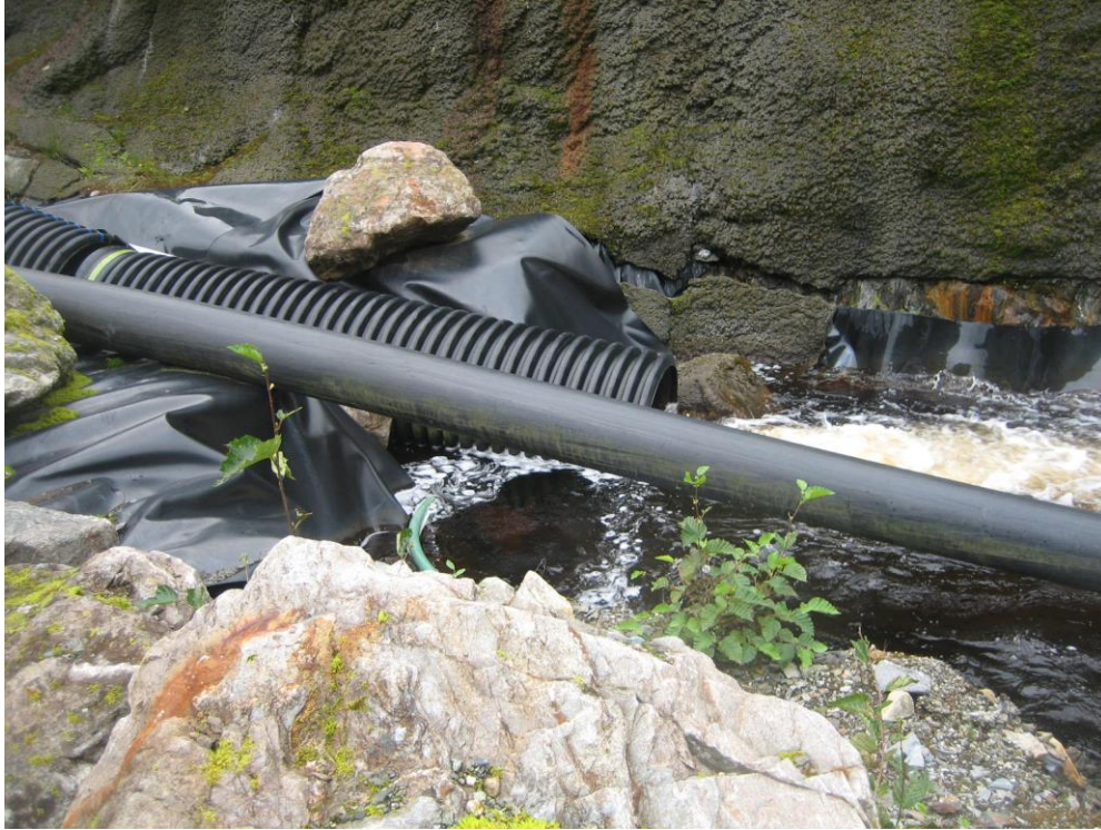
Photo G Diversion Outlet Pipes and lined channel below Lower Slate Lake Dam.
