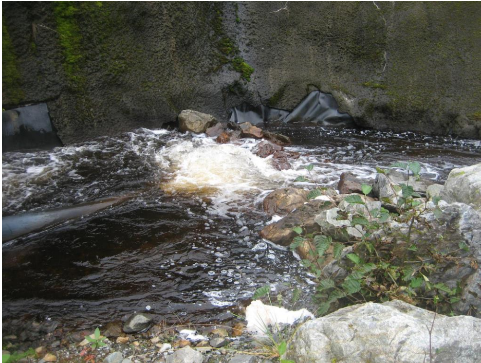
Photo F Diversion Outlet Pipes and lined channel below Lower Slate Lake Dam.
