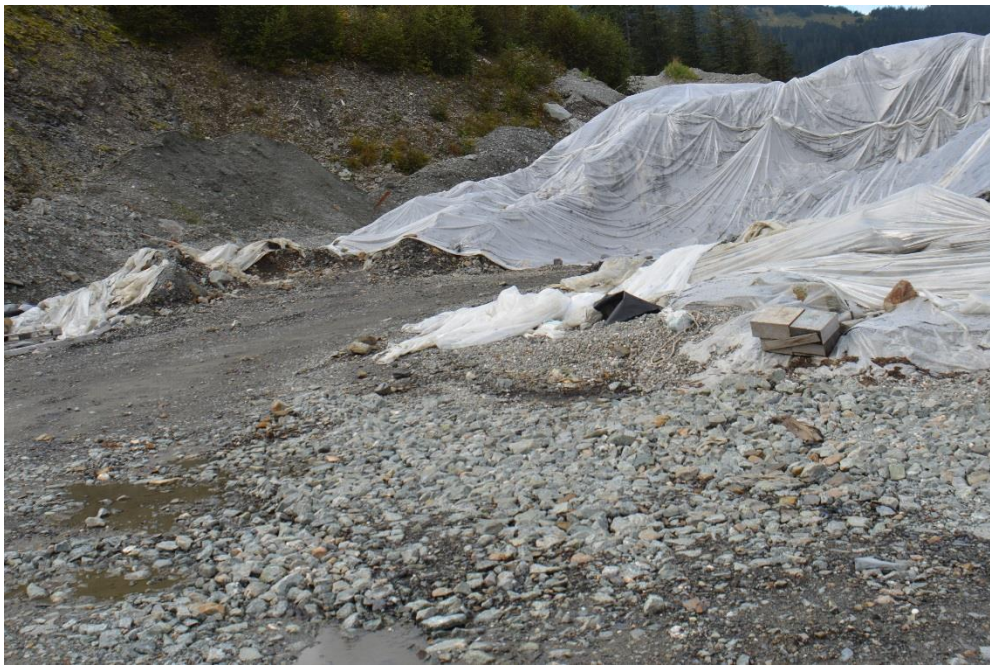
Photo JJ Pit 7 graphitic phyllite storage, missing a berm to capture runoff.
