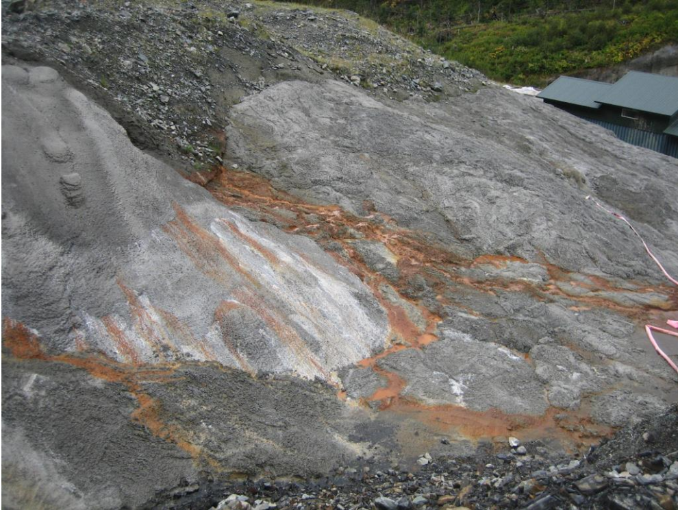
Photo U Lower Slate Lake Dam area downstream of east (left) abutment, shotcreted slopes (understood to have been excavated to rock) with staining from ARD seepage and collected seepage at toe of slope.
