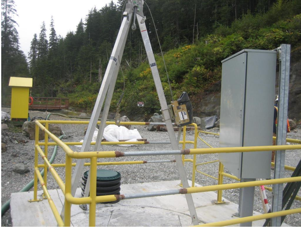
Photo II ARD seepage collection sump and seepage pump-back sump lift station (manhole) with sampling (safety) tripod and pump control panel, downstream of Dam.
