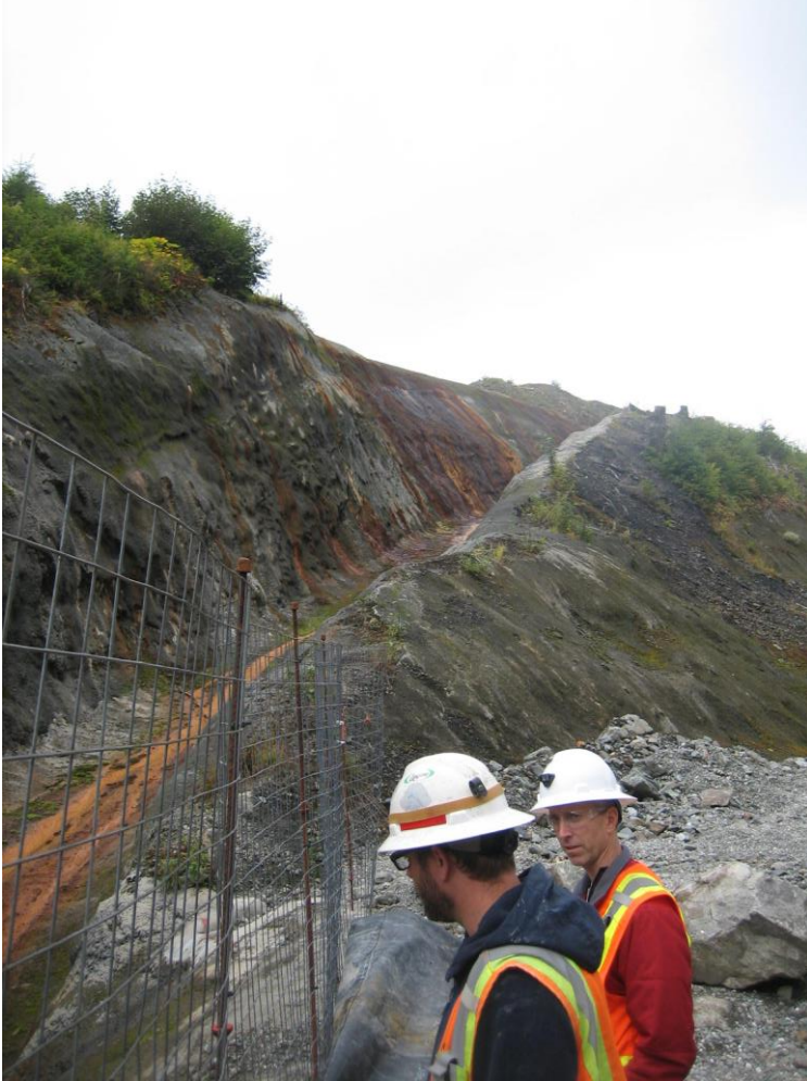
Photo DD Lower Slate Lake Dam collection channel along and downstream of west groin of dam below shotcreted west abutment wall.
