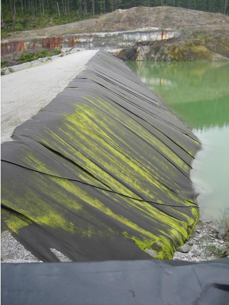
Photo R Lower Slate Lake Dam Stage 2 upstream slope with exposed geotextile, looking west.
