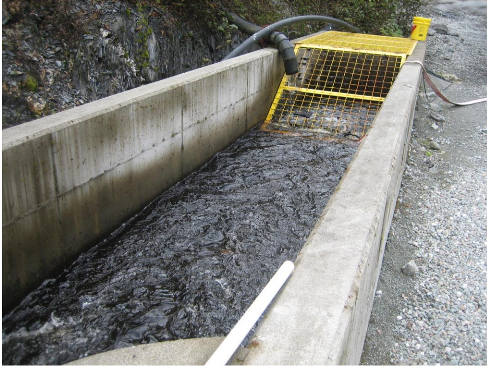
Photo O Parshall Flume for combined flow from Lower Slate Creek Diversion Dam & North Diversions at east (left) abutment of dam.
