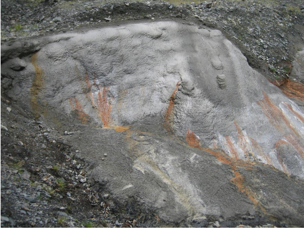
Photo T Lower Slate Lake Dam area downstream of east (left) abutment, shotcreted slopes (understood to have been excavated to rock) with staining from ARD seepage and collected seepage at toe of slope.
