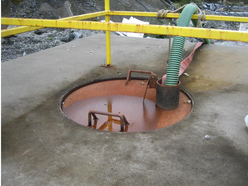
Photo AA Lower Slate Lake Dam Seepage Collection Sump.
