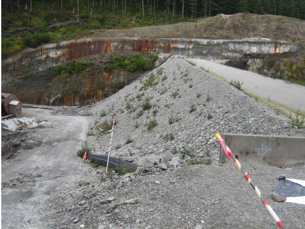
Photo S Lower Slate Lake Stage 2 Dam downstream slope and toe, looking west, Interim Spillway and west abutment wall in background
