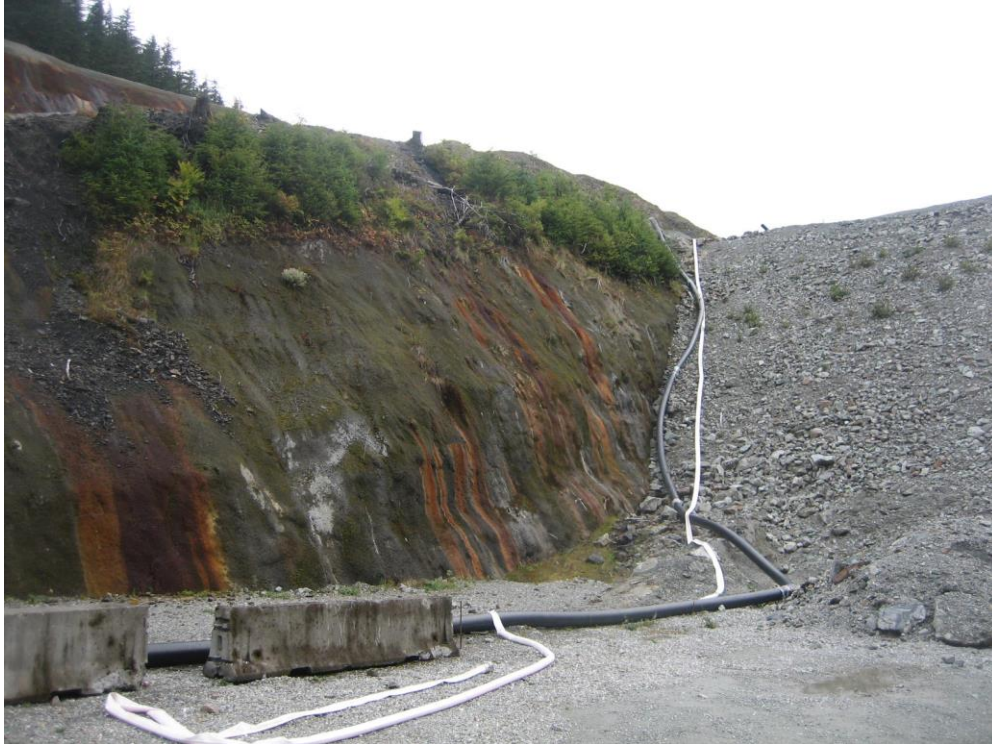
Photo W Lower Slate Lake Dam Stage 2 downstream slope. Seepage Collection Sump return pipeline along west groin of dam. Shotcrete west abutment wall with staining from ARD seepage.
