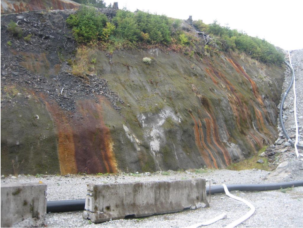
Photo CC Lower Slate Lake Dam Seepage Collection Sump return pipeline along west groin of dam. Shotcreted west abutment wall with staining from ARD seepage.
