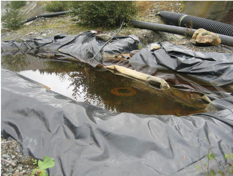
Photo HH Geomembrane-lined ARD seepage collection sump downstream of Lower Slate Lake Dam.
