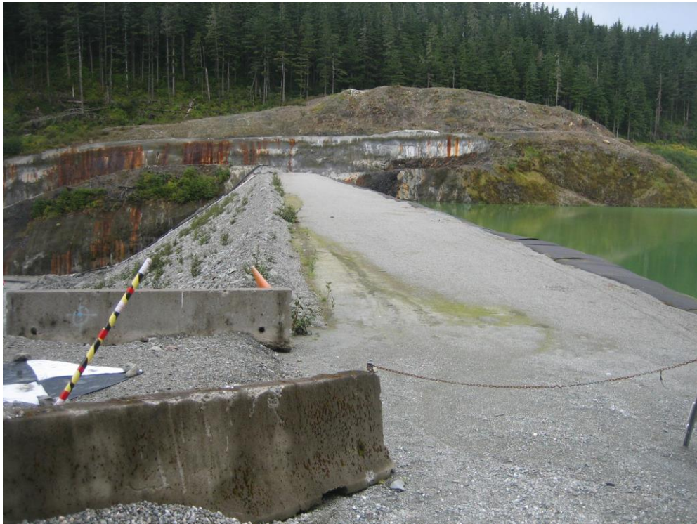
Photo P Lower Slate Lake Dam crest at Stage 2 elev. 715, Stage 2 Interim Spillway in background, looking west-southwest.
