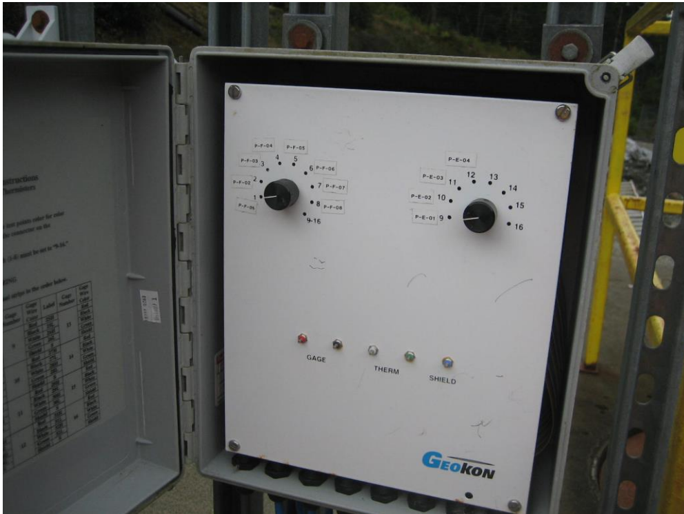
Photo X Lower Slate Lake Dam Vibrating Wire Piezometer readout panel/switchbox (located at Seepage Collection Sump).
