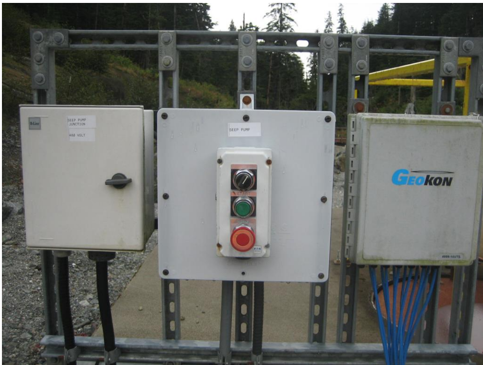
Photo BB Lower Slate Lake Dam Seepage Collection Sump control station, incl. Geokon vibrating wire piezometer readout panel.
