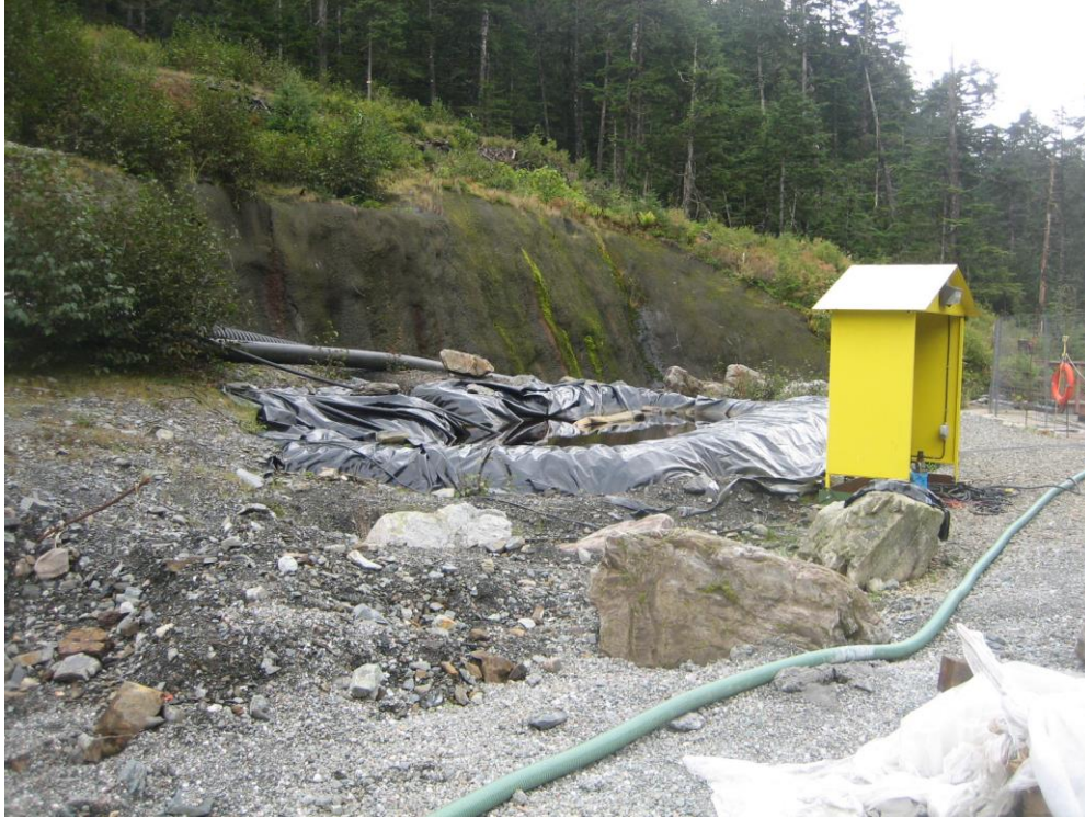
Photo GG Geomembrane-lined ARD seepage collection sump and ARD seepage pump-back sump lift station (manhole) with sampling (safety) tripod and pump control panel.
