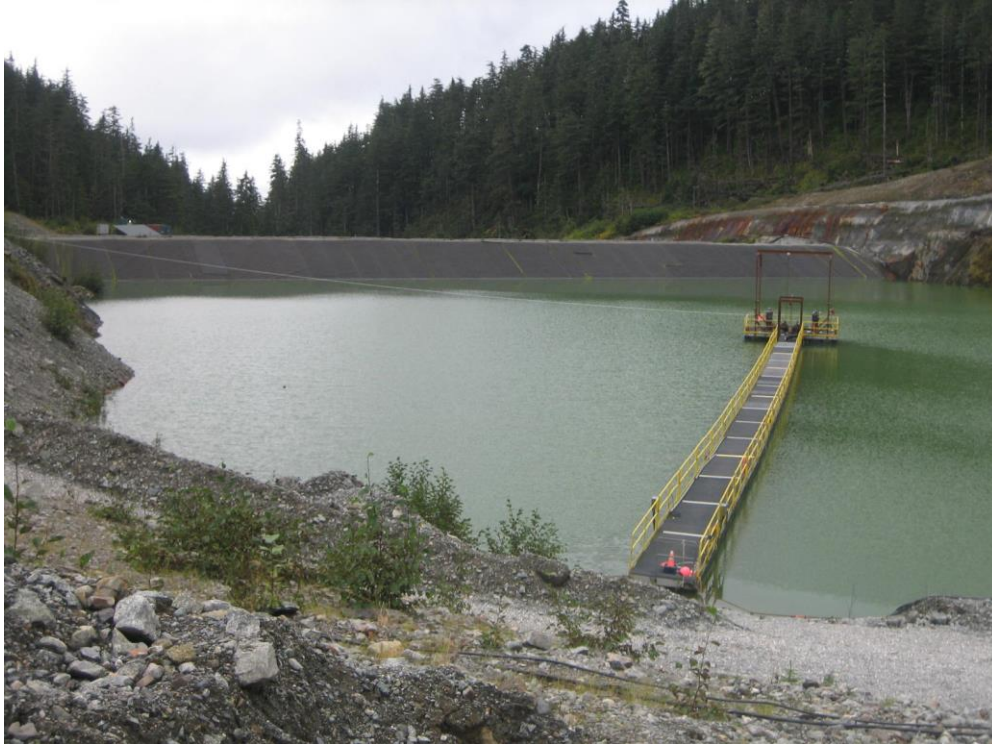
Photo K Lower Slate Lake Reclaim Water Line barge, Lower Slate Lake Dam upstream slope and Stage 2 Interim Spillway in background
