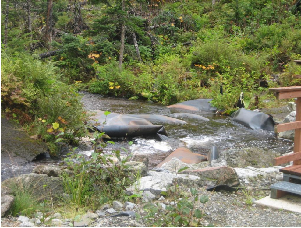
Photo E Diversion Outlet Pipes and lined channel below Lower Slate Lake Dam.
