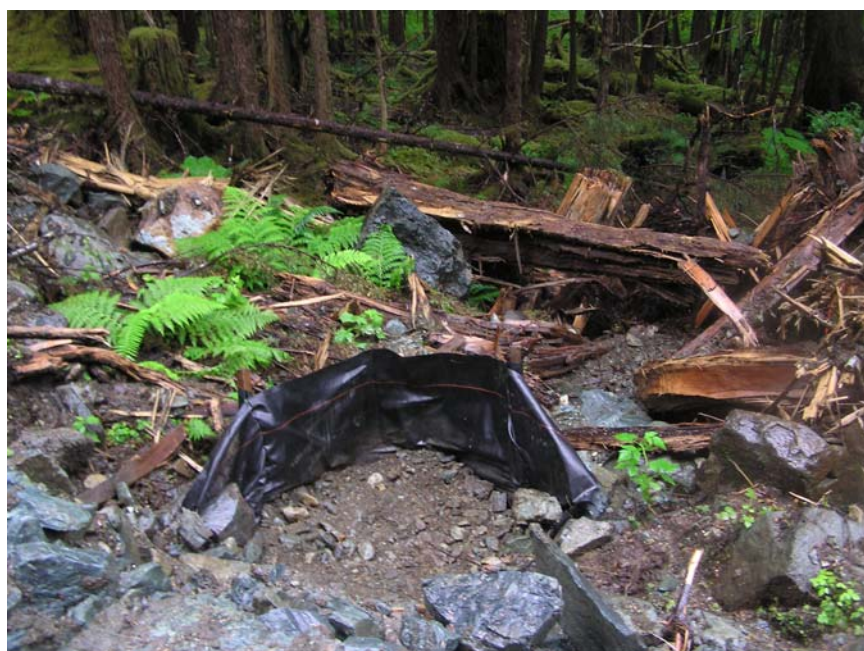
Sediment trap along road
