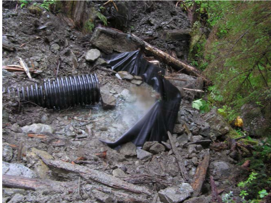
Sediment trap along road
