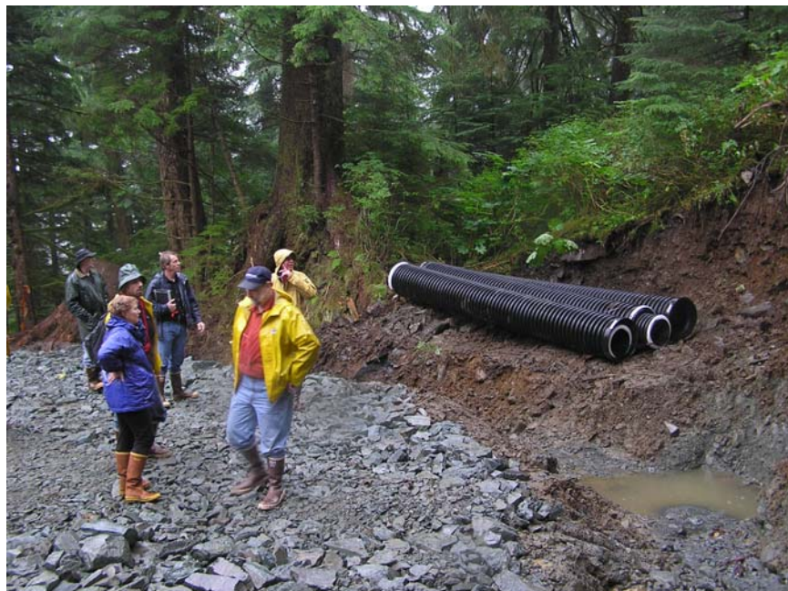
Where road to NAG rock dump will leave the portal access road
