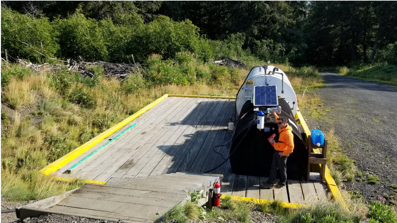
Photo 1. Fuel Station at the Glacier Creek Laydown. Tanks were emptied and winterized in October 2019, unused in 2020.
