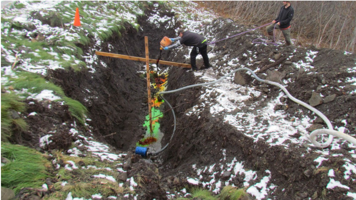
Figure 7. Fluorescein dye introduction at Trench T-1. Note blue water diffuser in bottom of trench.
