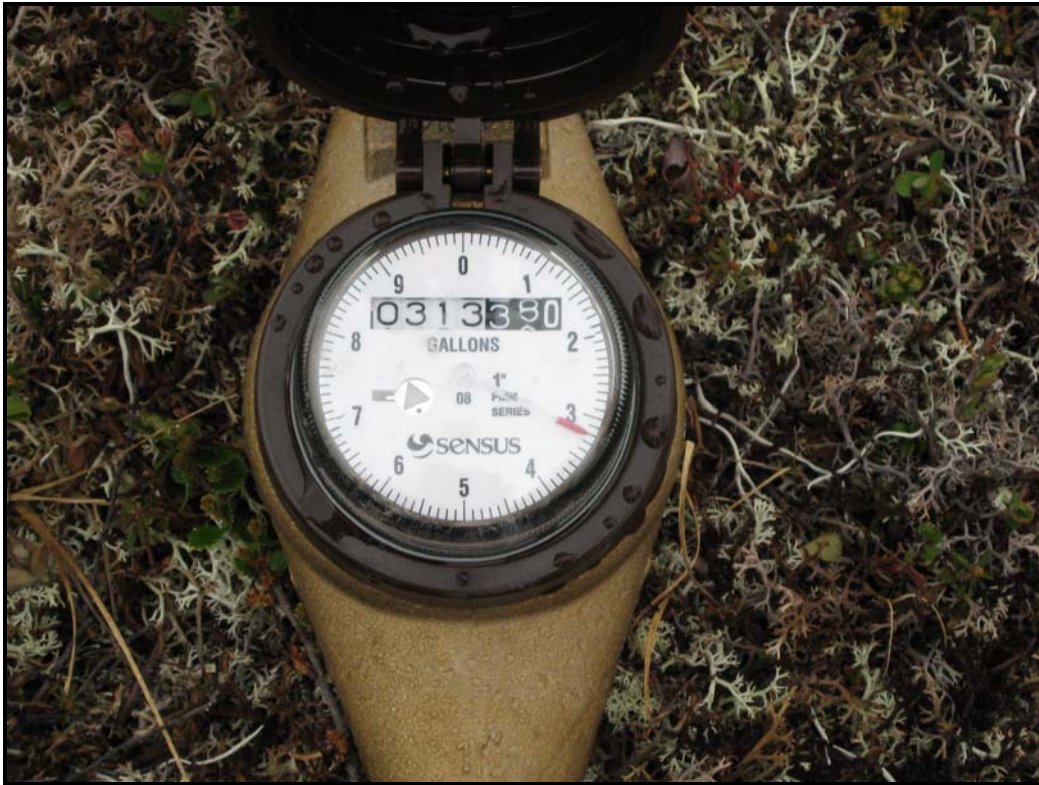
Figure 5. New totalizer that PLP is using to track water usage. During site visit, pumping rate was estimated at 20 gpm.
