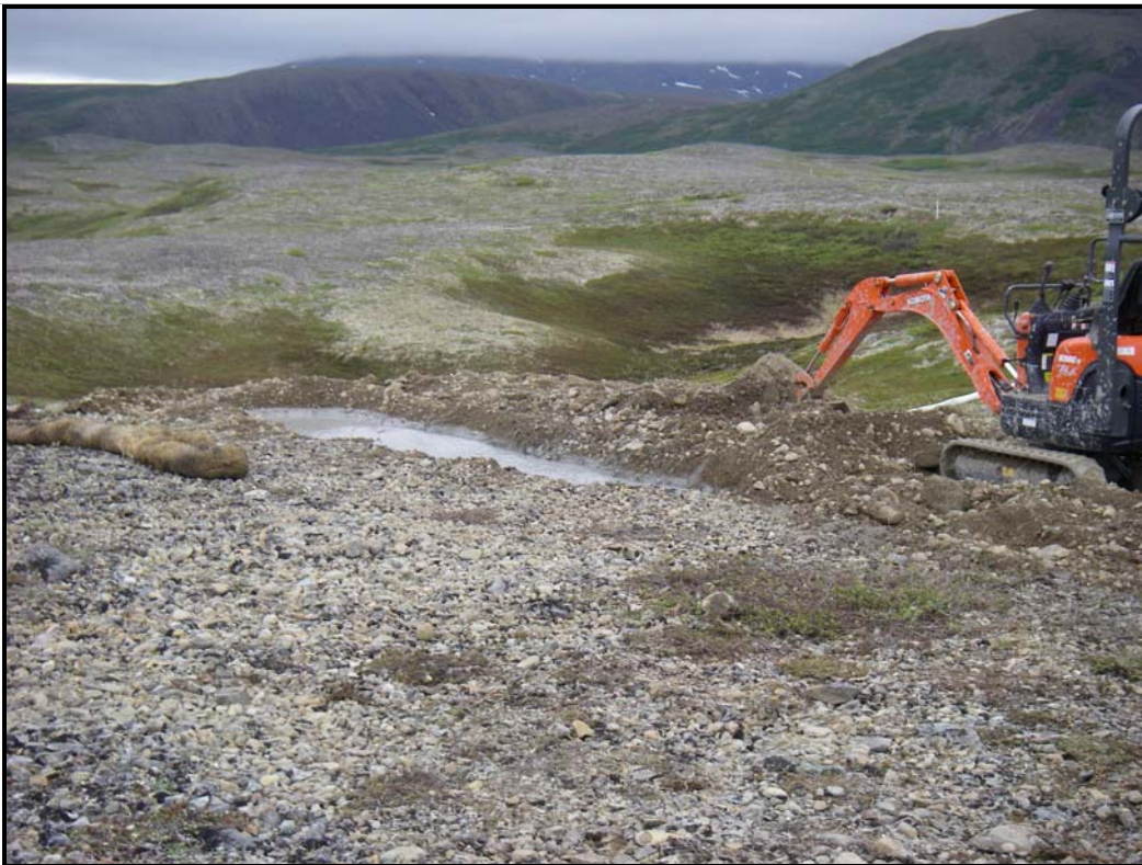
Figure 20. The drill rig was recently removed from this site and the sump pits are being filled in as the beginning stage of reclamation.
