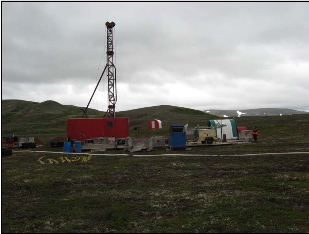
Figure 1. Drill Rig #3 on DH 10480. Note tundra pads, fuel containment and oil scrubbers (blue barrels).
