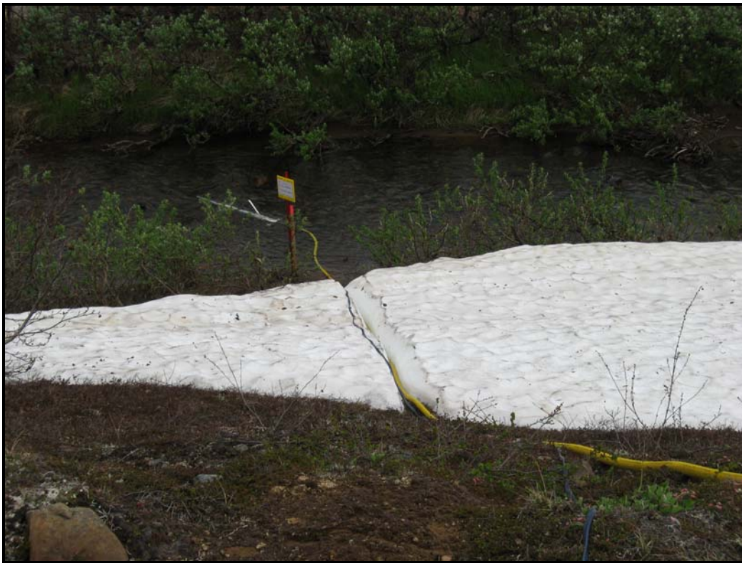
Figure 6. Water intake line extended from the upland down to the creek. Pump is visible in the water, as well as required sign indicating this is a water take location.
