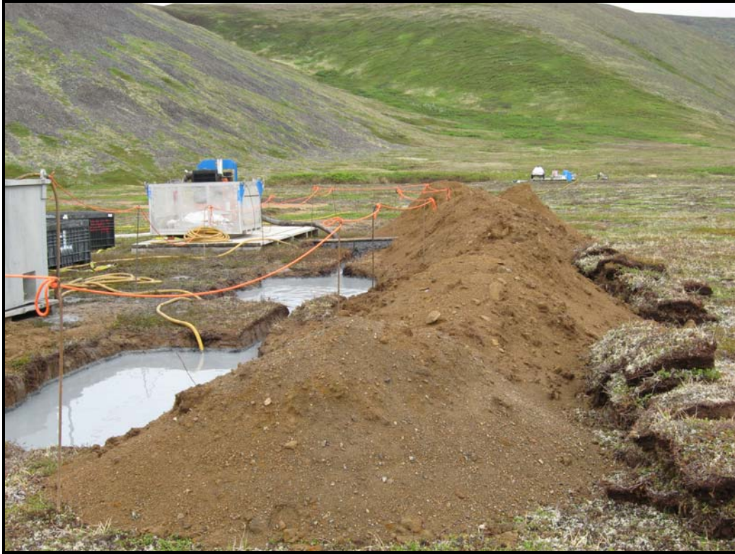
Figure 3. Sump pits (on left) and tundra stock pile being saved for reclamation (on right).
