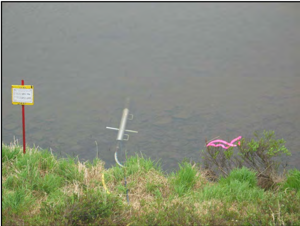
Photo #6. Submersible pump in Frying Pan Lake.
