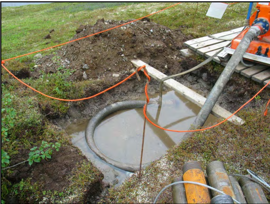
Photo #4. Mud sump.
