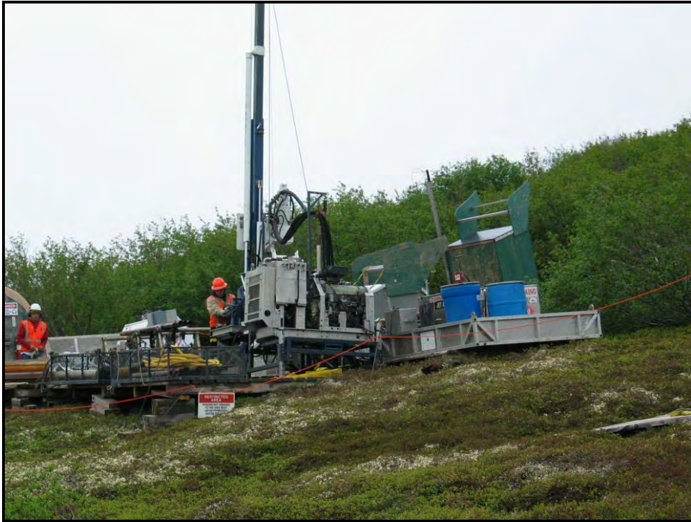
Photo #1. Drill Rig #4 on CH12-297. Note Blue hydrocarbon scrubber barrel and blue sorbent pad barrel, both in aluminum secondary fuel containment.
