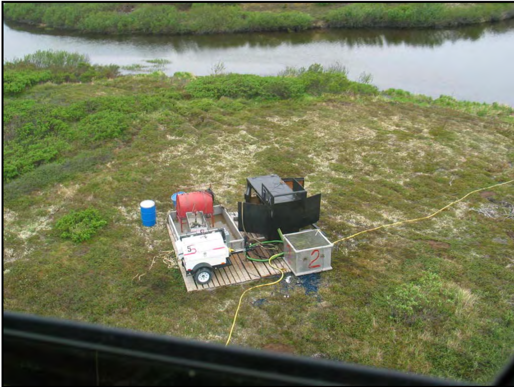
Photo #5. Generator and fuel for submersible water pump. Blue barrels are sorbent pads and scrubber barrel.
