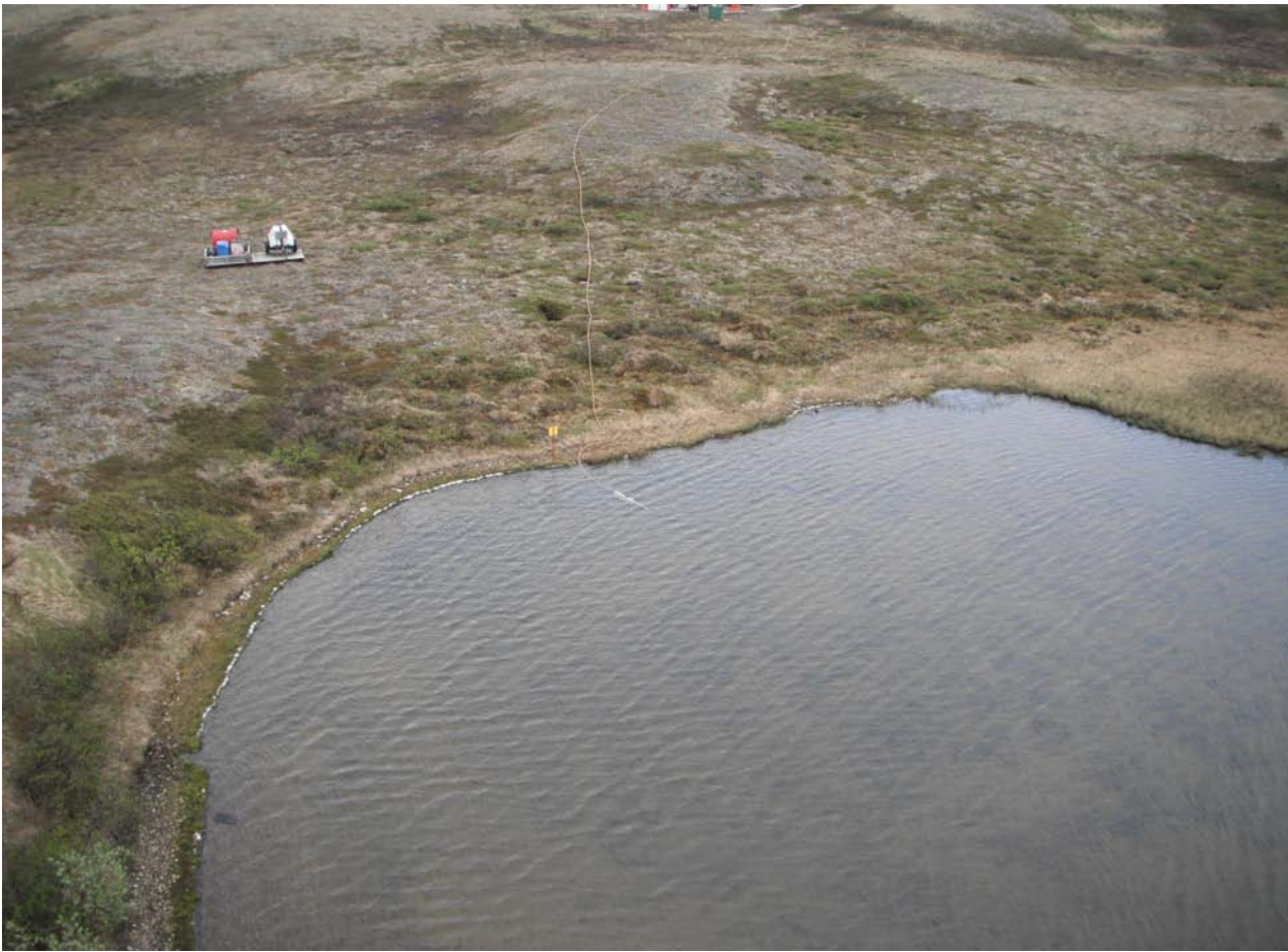
Figure 10 – GH 11235 Water Source and Pump – Set-up not complete
