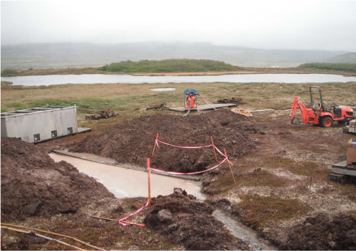
Figure 3 – Drill Hole 11533 Sump Pit, Recirculation Tank, and Discharge Pump
