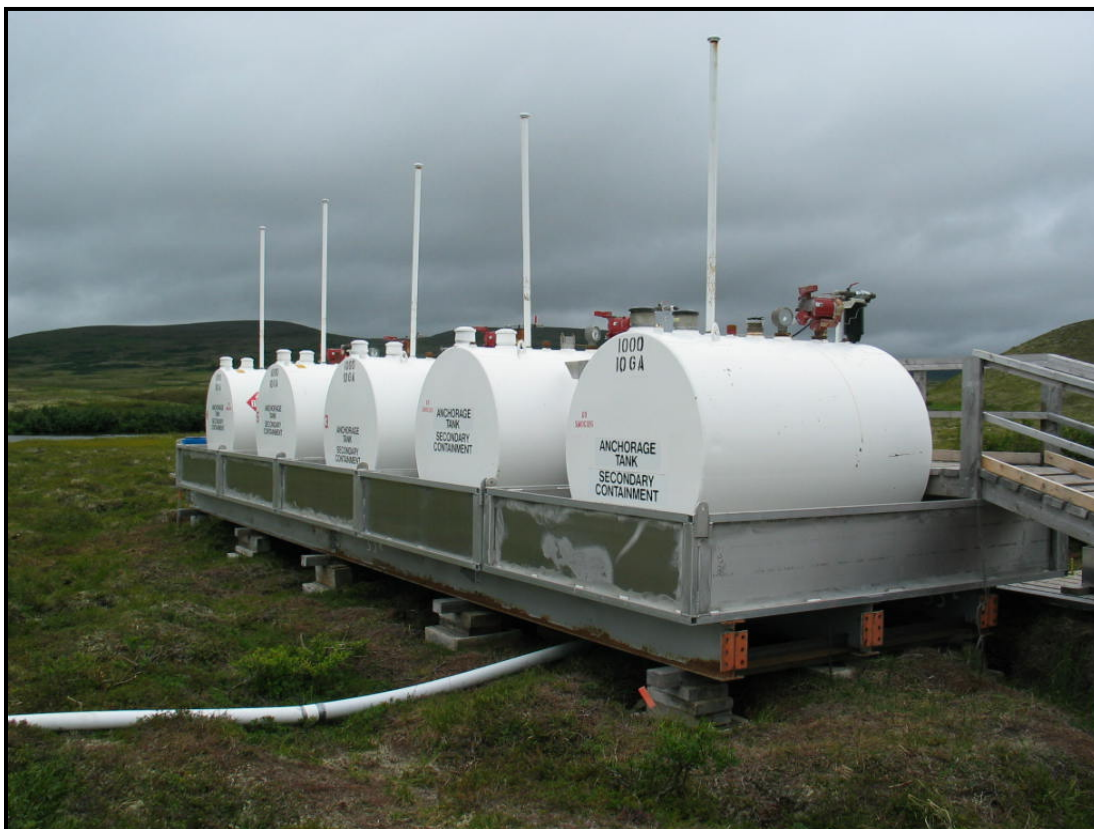
Figure #1. Fuel Storage and Secondary Containment at Big Wiggly Lake
