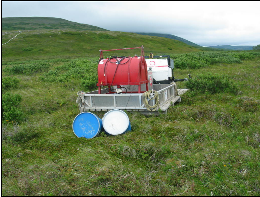
Figure #10. Water pump for DDH 10498. Note fuel containment, scrubber barrel, and spill kit.
