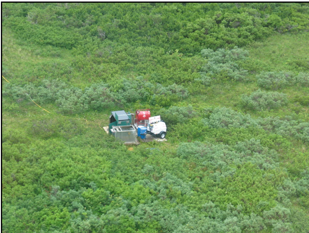
Figure #7. Water pump for DDH 10947. Note fuel containment, spill kit, and scrubber barrel.
