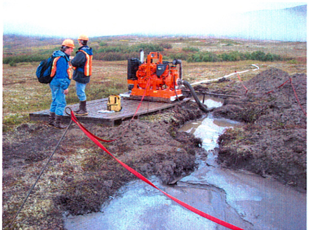
Figure 4. Series of three sump pits with Godwin pump and discharge to uplands.
