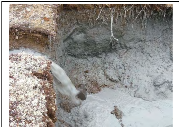
Outfall to sump pit #3, beginning to refill.
