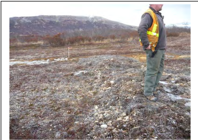
Mounded soil filling recirculation trenches.
