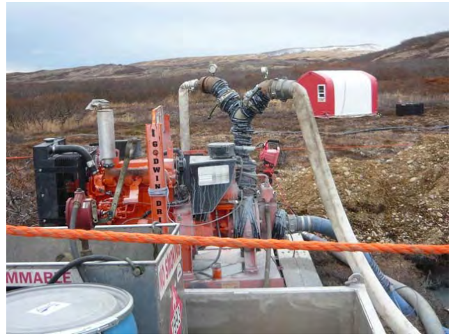
Recirculation tank, three compartments full, one empty.
