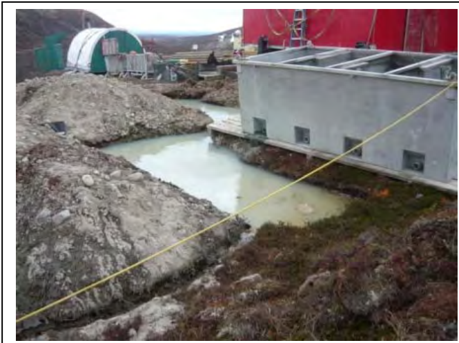
Upper sump pits, empty recirc. tank, DDHH 11541.
