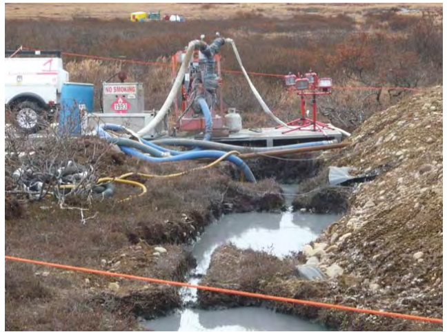
Sump trenches 4&5, Godwin redistribution pump.
