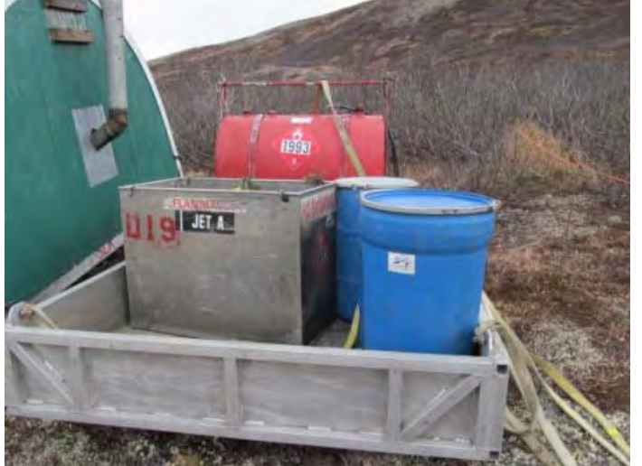
Fuel containment and cleanup kits by warming hut.
