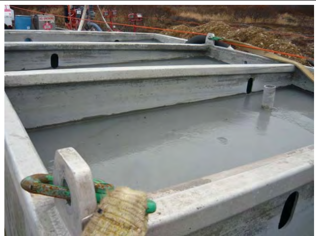
Recirculation tank, three compartments full, one empty.
