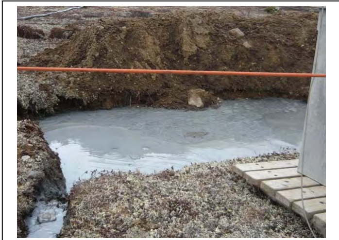
Recirculation water flow filling sump pit #1.
