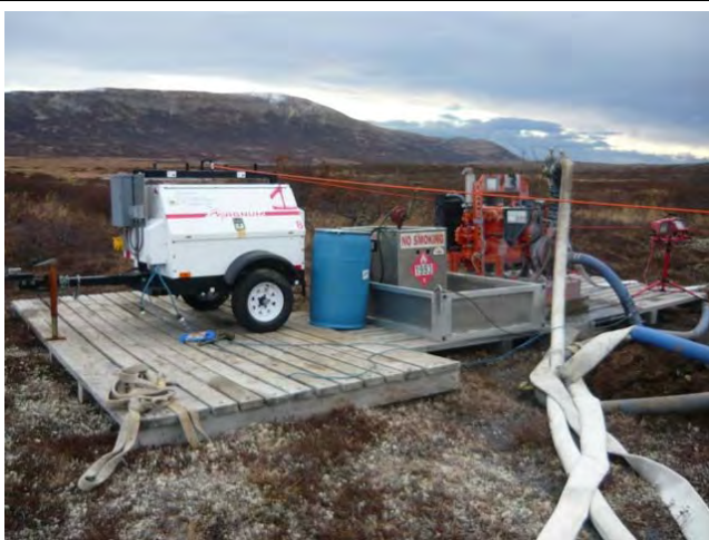
Godwin pump platform, fuel containment, generator.
