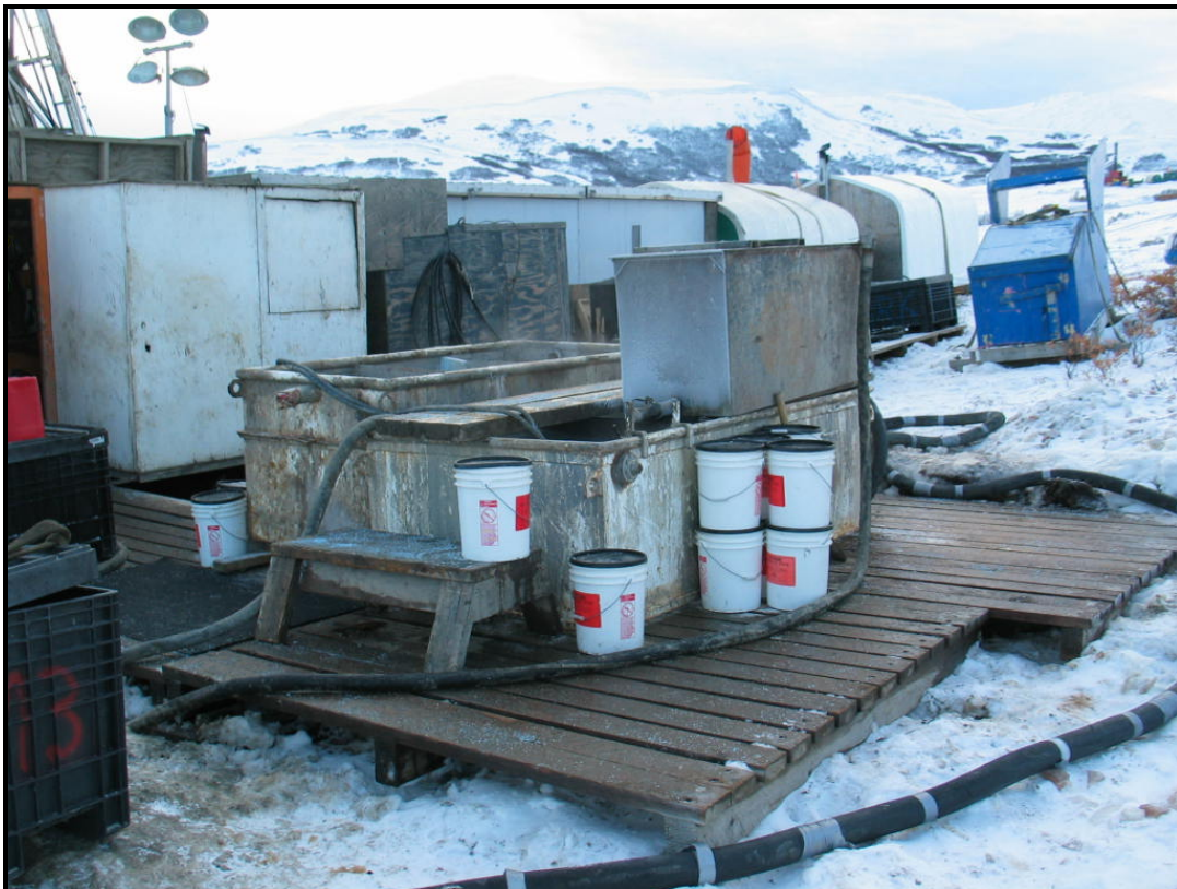
Photo #6. Recirculation mud tank on drill #1.
