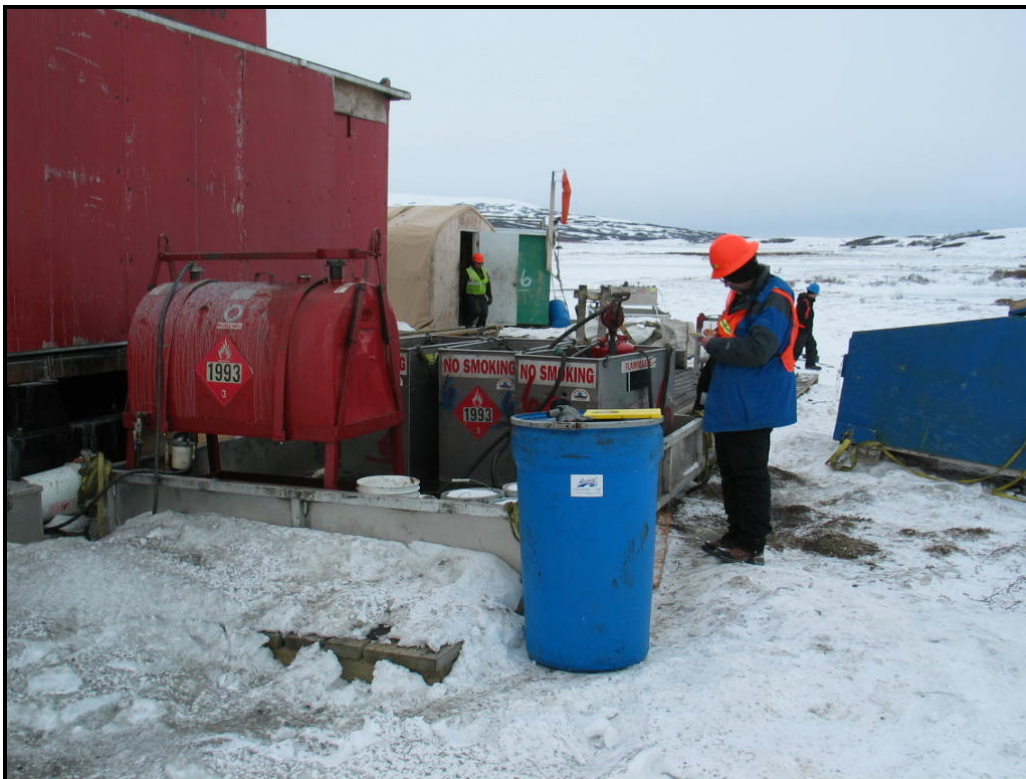
Photo #30. Fuel containment at drill #6.
