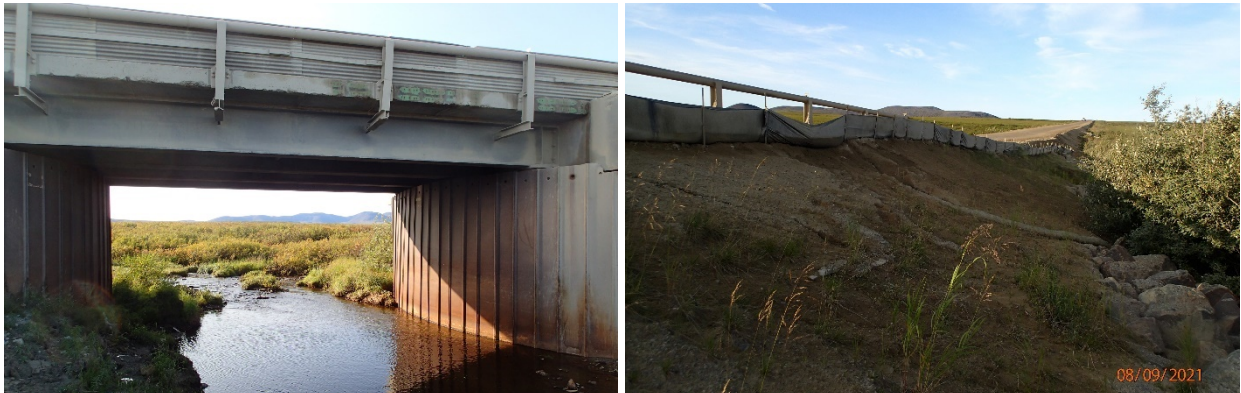
Figure 5. The bridge over Little Creek with metal sheeting in place to prevent road runoff on the bridge (left), and silt fencing directing runoff away from Anxiety Ridge Creek (right).
