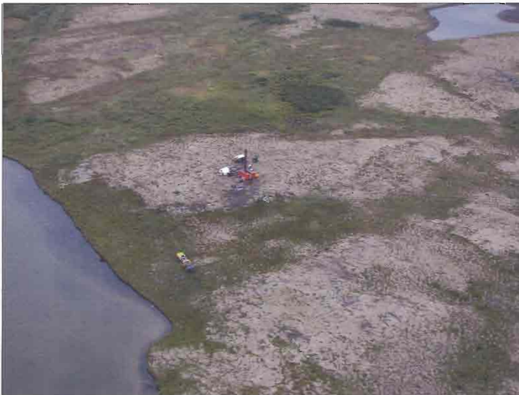
Water supply generator and submersible pump
