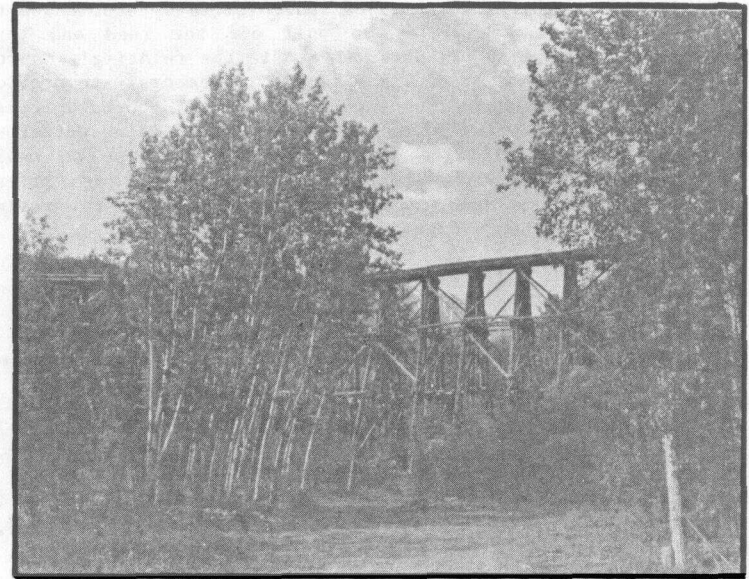
The Gilahina trestle, viewed from the small parking area near the road crossing of the Gilahina River. This is an important visual and historical landmark which needs restorative work.
