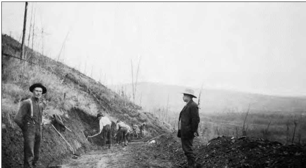
Figure 19. Excavating by hand on the Richardson Highway, 1914. Source: Archives, University of Alaska, Fairbanks.
