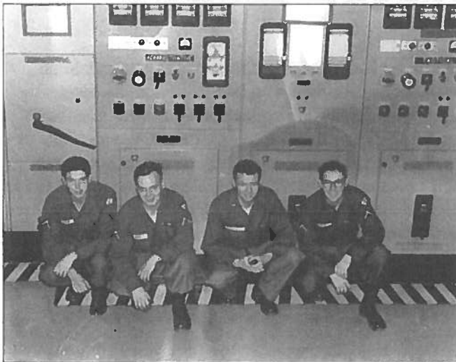
Figure 24: Personnel in front of 250 kW generator control panels. Courtesy Ralph New.
