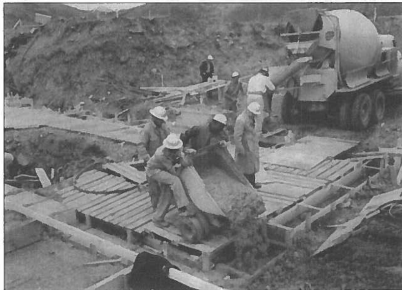
Figure 5: Construction workers pouring concrete ---Site Summit. National Archives and Records Administration. RG 77.
